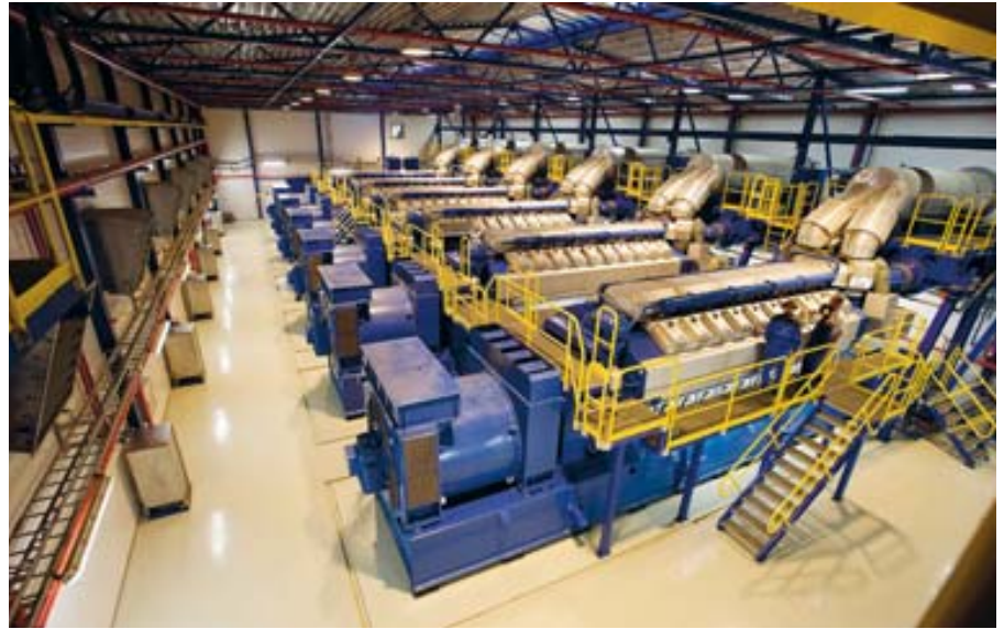
■ Fig. 11 – High resistance grounding cubicles installed against the wall opposite to the generators in a power plant.
