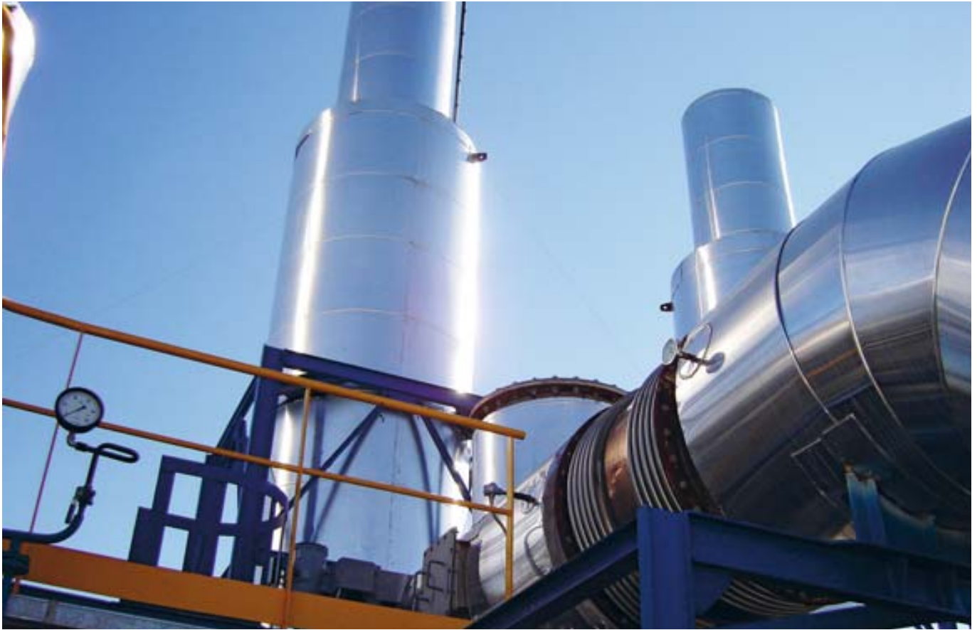
■ Fig. 2 – The integrated oxi installed in a power plant in Turkey.
