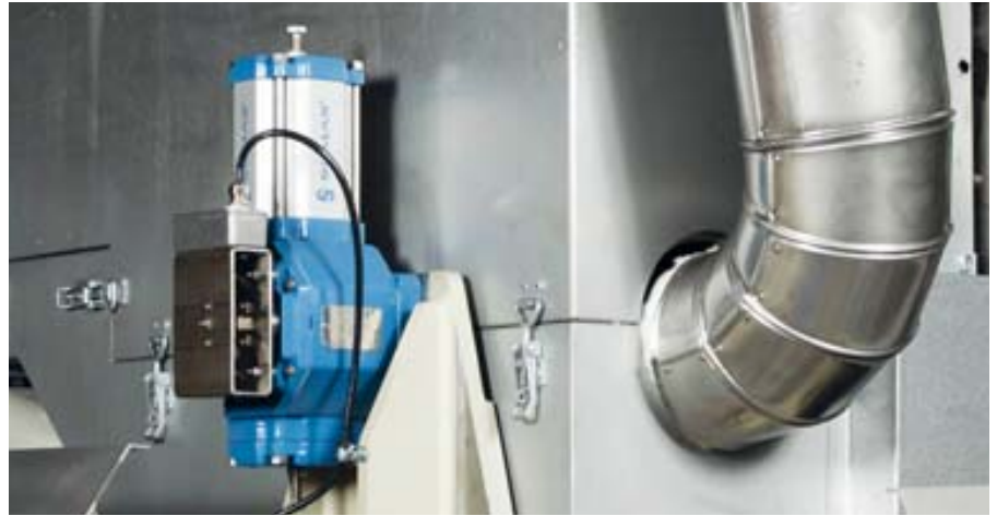
■ Fig. 3 – The electro-pneumatic waste gate for air-fuel ratio control.
