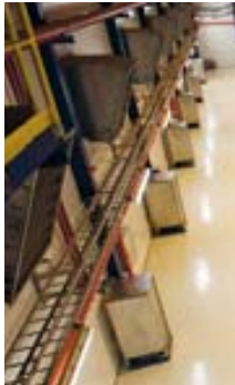
High resistance grounding combines the equipment friendliness of the ungrounded system, while still providing control of transient and temporary voltage (more on page 27).
