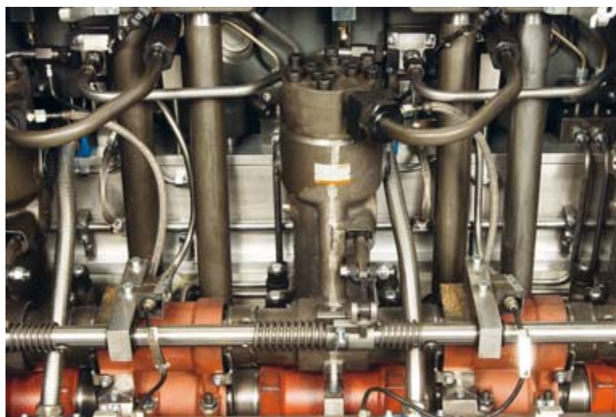
■ Fig. 6 – Camshaft driven injection pump for back up fuel.
