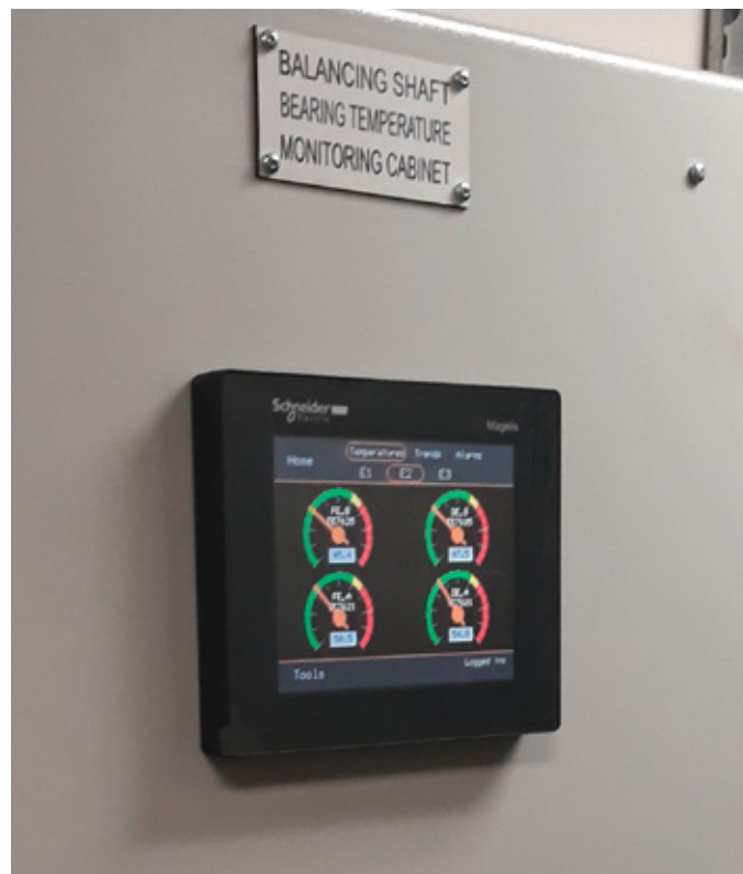
The monitoring cabinet is an integral part of the temperature monitoring system.
