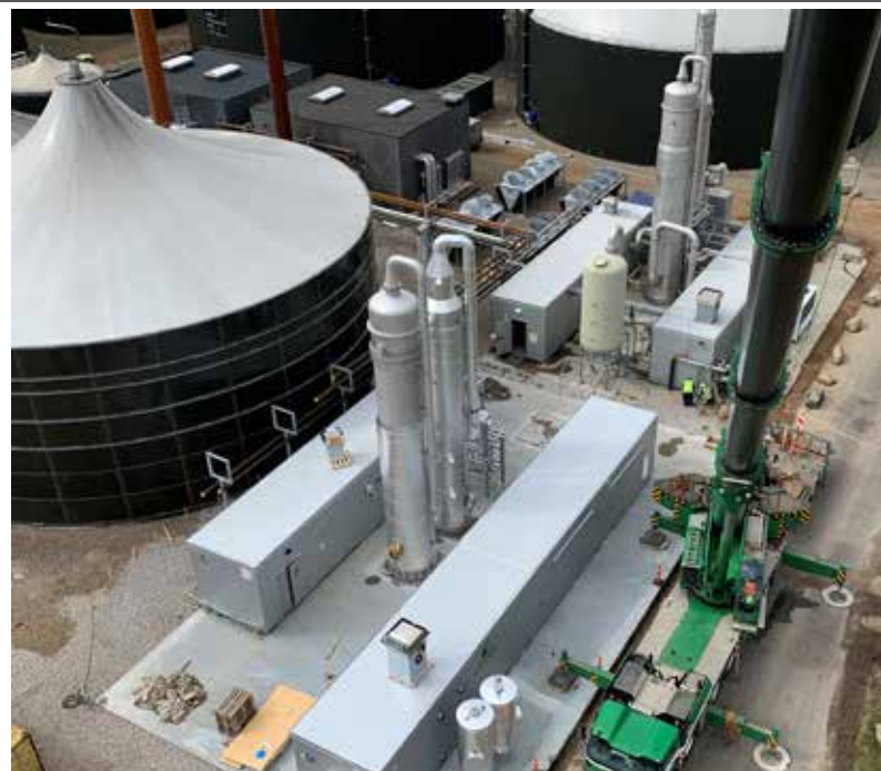
Sönderjysk biogas upgrading plant in Denmark with two Wärtsilä biogas upgrading plants model Puregas CA80, upgrading 10,000 Nm 3 /h of biogas
