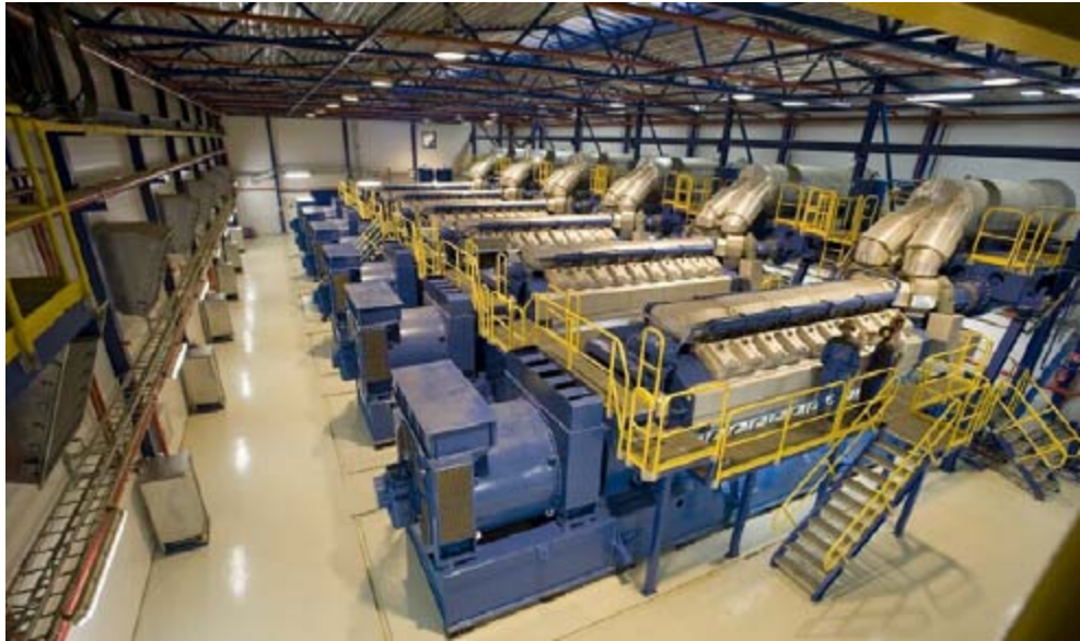
View inside a combustion engine power plant engine hall.
