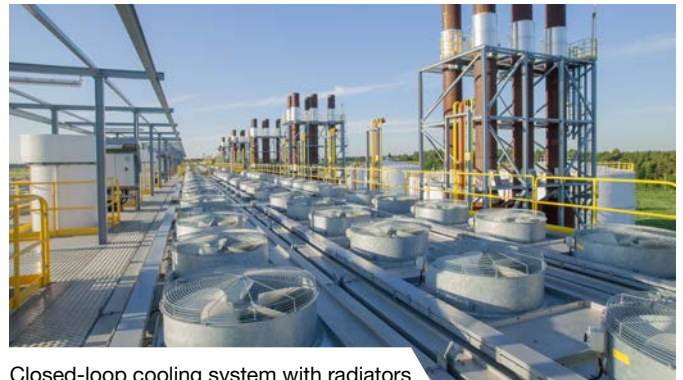
Closed-loop cooling system with radiators
