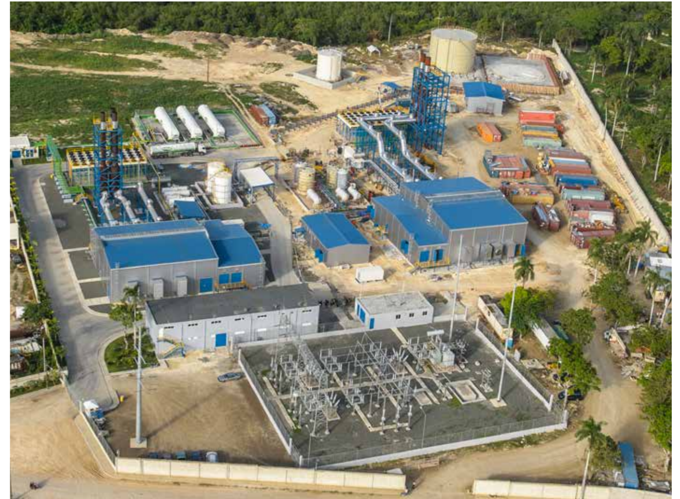
■ Fig. 10 - LNG satellite terminal for a 59 MW Wärtsilä dual-fuel power plant in the Dominican Republic. Note the truck unloading LNG to the LNG bullet tanks in the top left corner.
