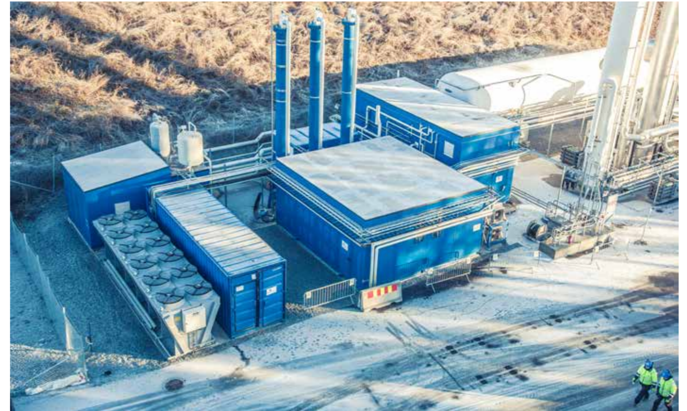
■ Fig. 8 - EGE Biogas 4000 TPA biogas-to-LNG plant in Norway, Design and equipment delivery 2014 by Wärtsilä is an example of a Mini LNG liquefaction plant.
