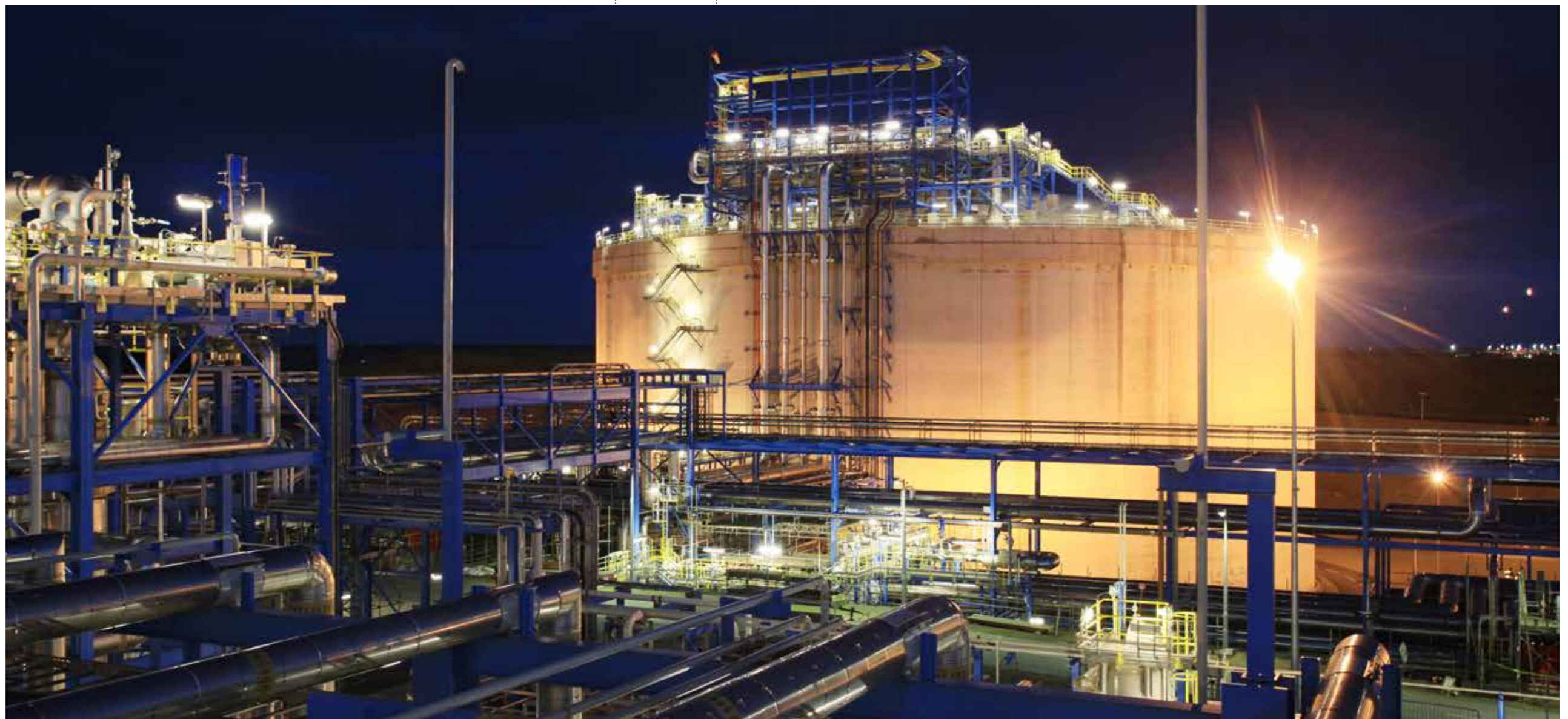
■ Fig. 14 - Dragon LNG Terminal, in Wales, UK. Wärtsilä will deliver the re-liquefaction system, to be installed during 2016–17. Photo: Dragon LNG Limited.
