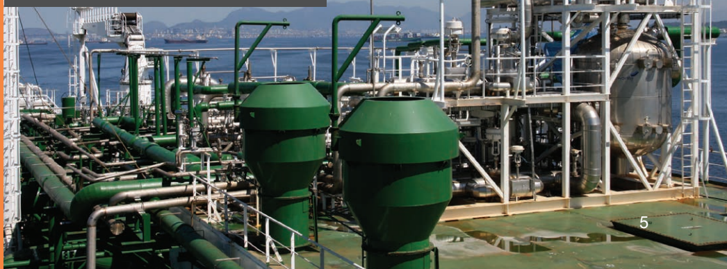
Wärtsilä Hamworthy regasification system on trial onboard LNG FSRU vessel 'Golar Winter'
