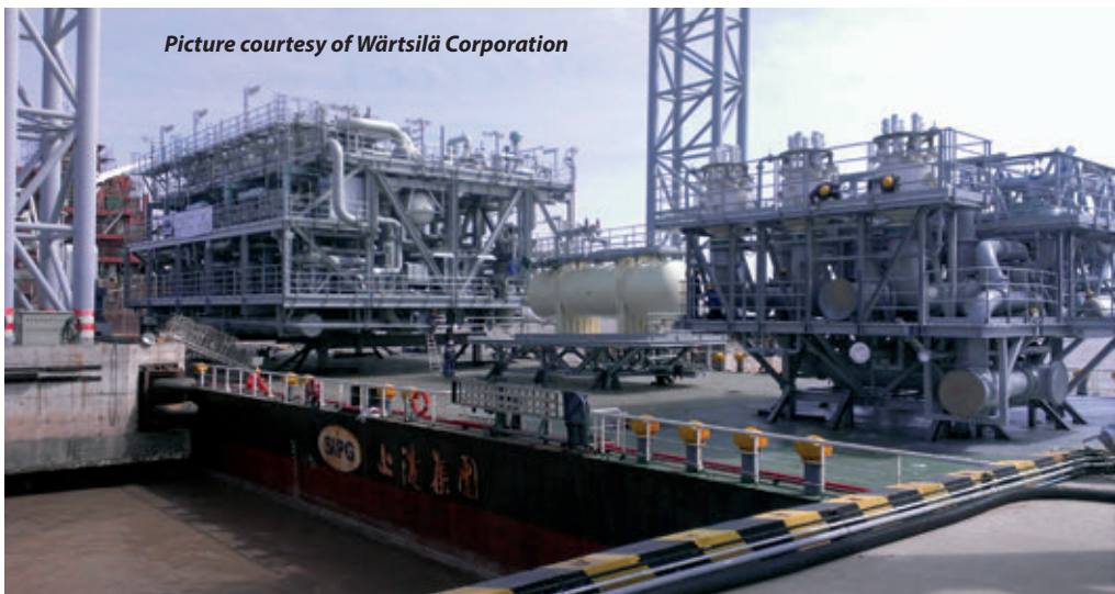
Wärtsilä Hamworthy regasification modules for Hoeg 170,000m 3 FSRU
