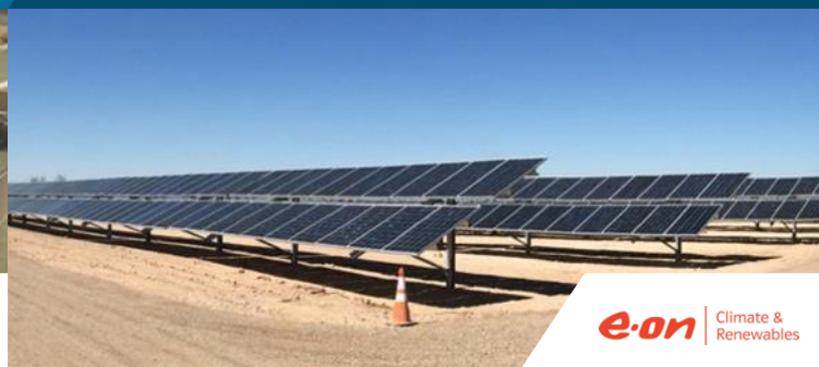
10MW Solar Integration AZ, USA
