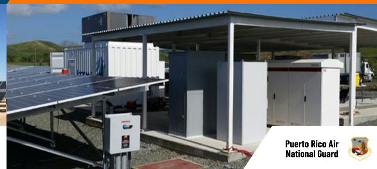
1MW Solar Micro grid Puerto Rico, USA
