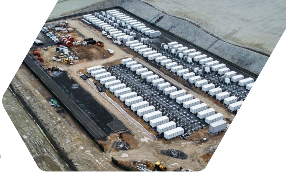
Aerial view of Zenobē's 200 MW / 400 MWh battery energy storage site in construction in Blackhillock, Scotland © Zenobē
