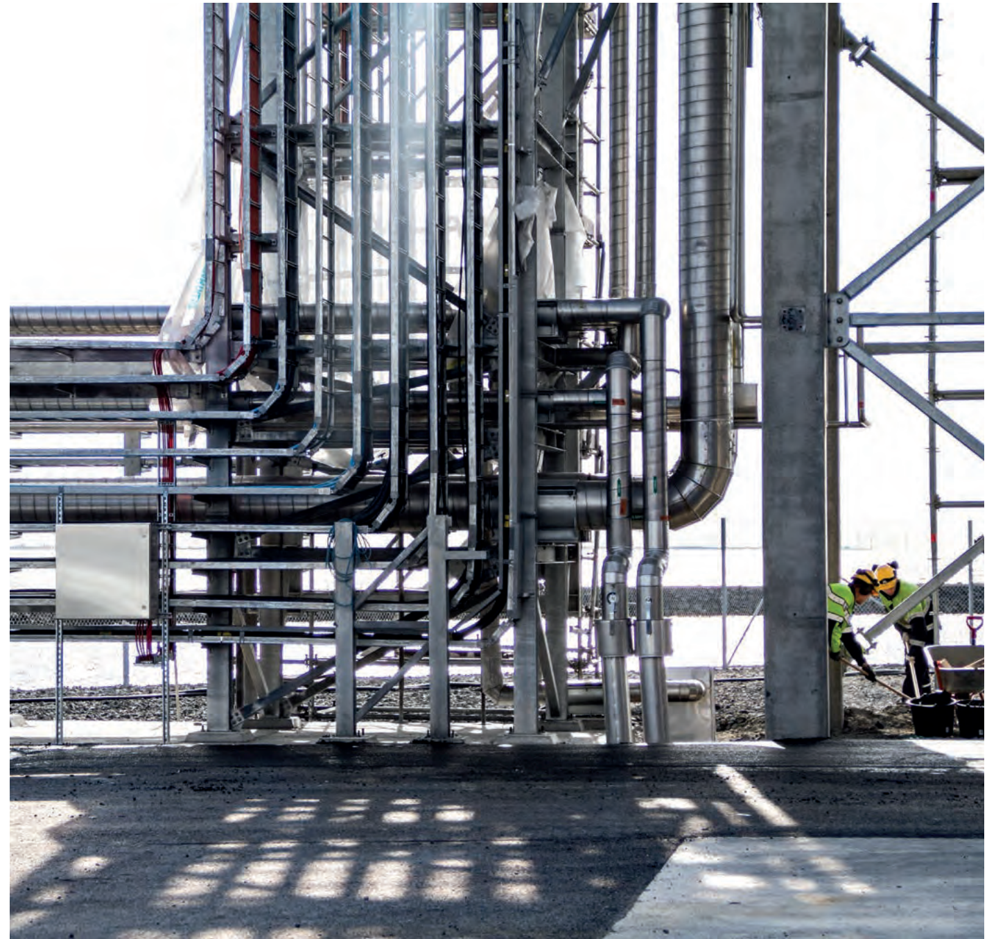
Wärtsilä was a pioneer in liquefied natural gas (LNG) transport. At the place of use, the liquefied natural gas is vaporised into gas.
