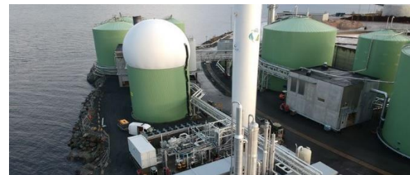
5 Wärtsilä builds major plant for the production of REEFUEL, climate-neutral Bio-LNG
