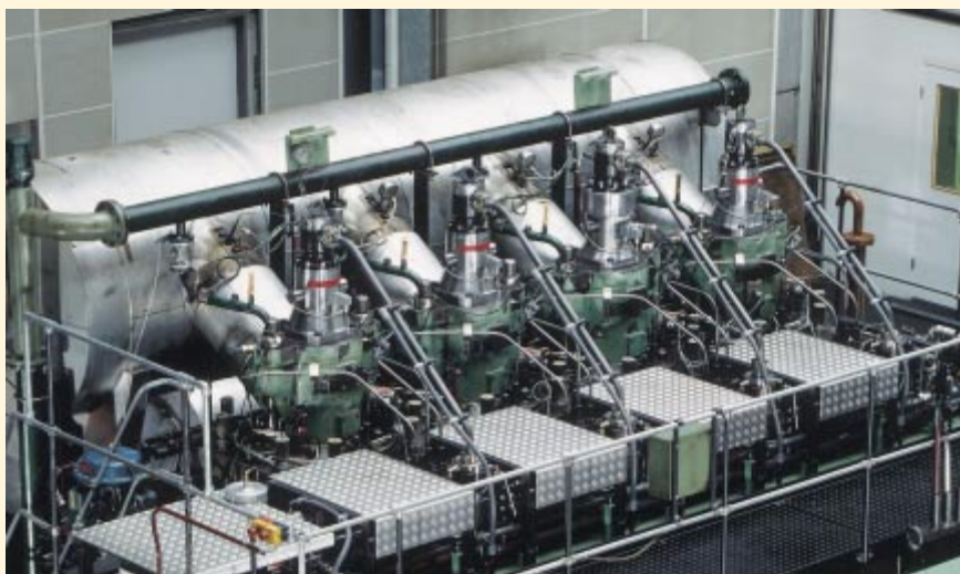
The four-cylinder Sulzer RT-flex58T-B research engine has been running in the Diesel Technology Center, Winterthur, since June 1998. In the long series of research and reliability tests, the common rail system has proven that it will operate on the same grades of heavy fuel oil as the "classic" Sulzer RTA-series engines. ■
