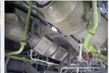
Exhaust gas cleaning
