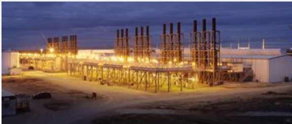
South Texas Electric Cooperative, USA
