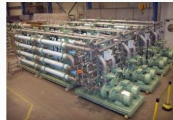
Waste & fresh water management
