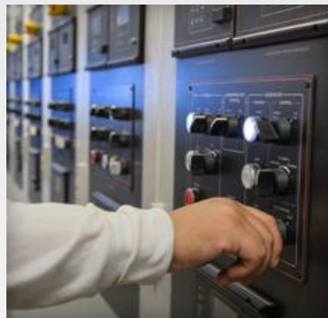
Electrical and automation services
