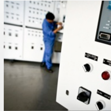
Electrical & Automation services
