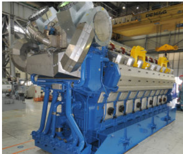
4.2. Wärtsilä contracted to supply a 220MW natural gas fuelled power plant in Oregon, USA, to accommodate rapidly changing input levels of renewable energy sources to the grid.
