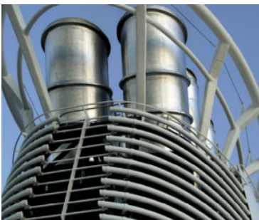
29.10. The first Wärtsilä closed loop scrubber, installed on Containership VII, received a compliance certificate.
