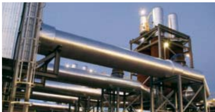
SCR reactors at Barrick Western power plant.
