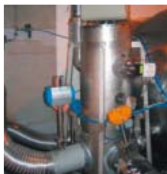
New time-shared emission measuring equipment during testing.
