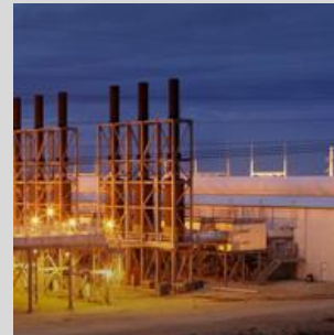
Flexible grid stability power plants
