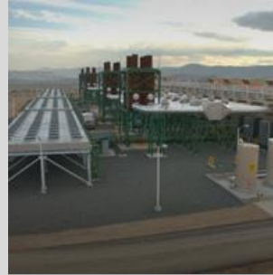
Grid stability and peaking
