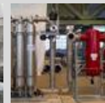
Inert gas systems
