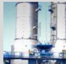
Flue gas desulphurisation & scrubbers
