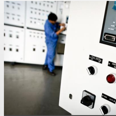
Electrical & automation services
