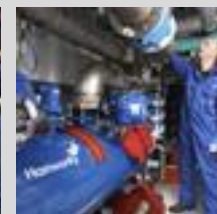
Ballast water system
