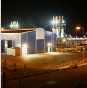
Flexible base-load power generation
