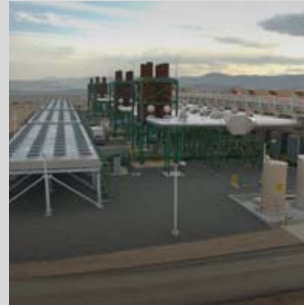
Grid stability and peaking
