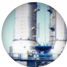
Flue gas desulphurisation & scrubbers
