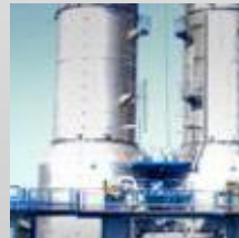
Flue gas desulphurisation & scrubbers
