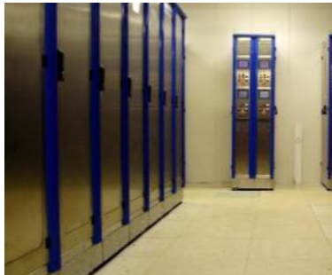
Power Electric Systems
