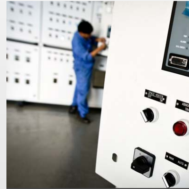
Electrical & automation services
