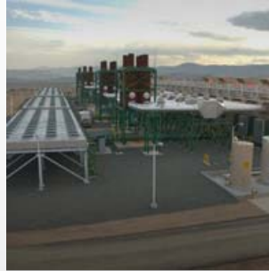
Grid stability and peaking
