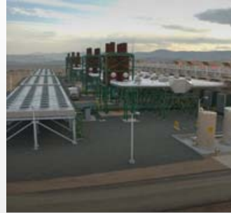
Grid stability and peaking
