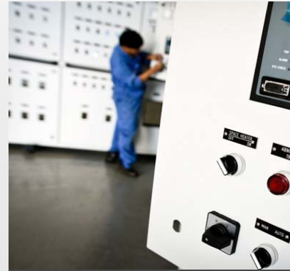
Electrical & automation services
