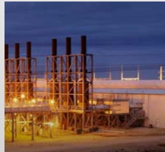
Flexible grid stability power plants
