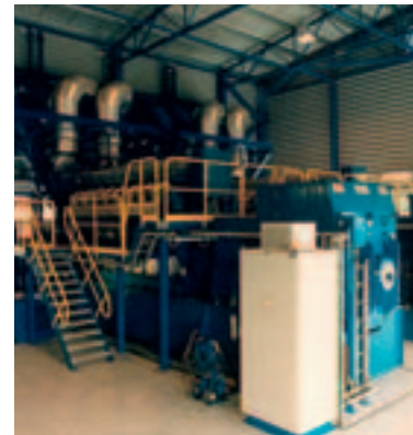
The two Wärtsilä 18V32GD engines in the Dygoil plant in Ecuador use the fuel sharing principle.
