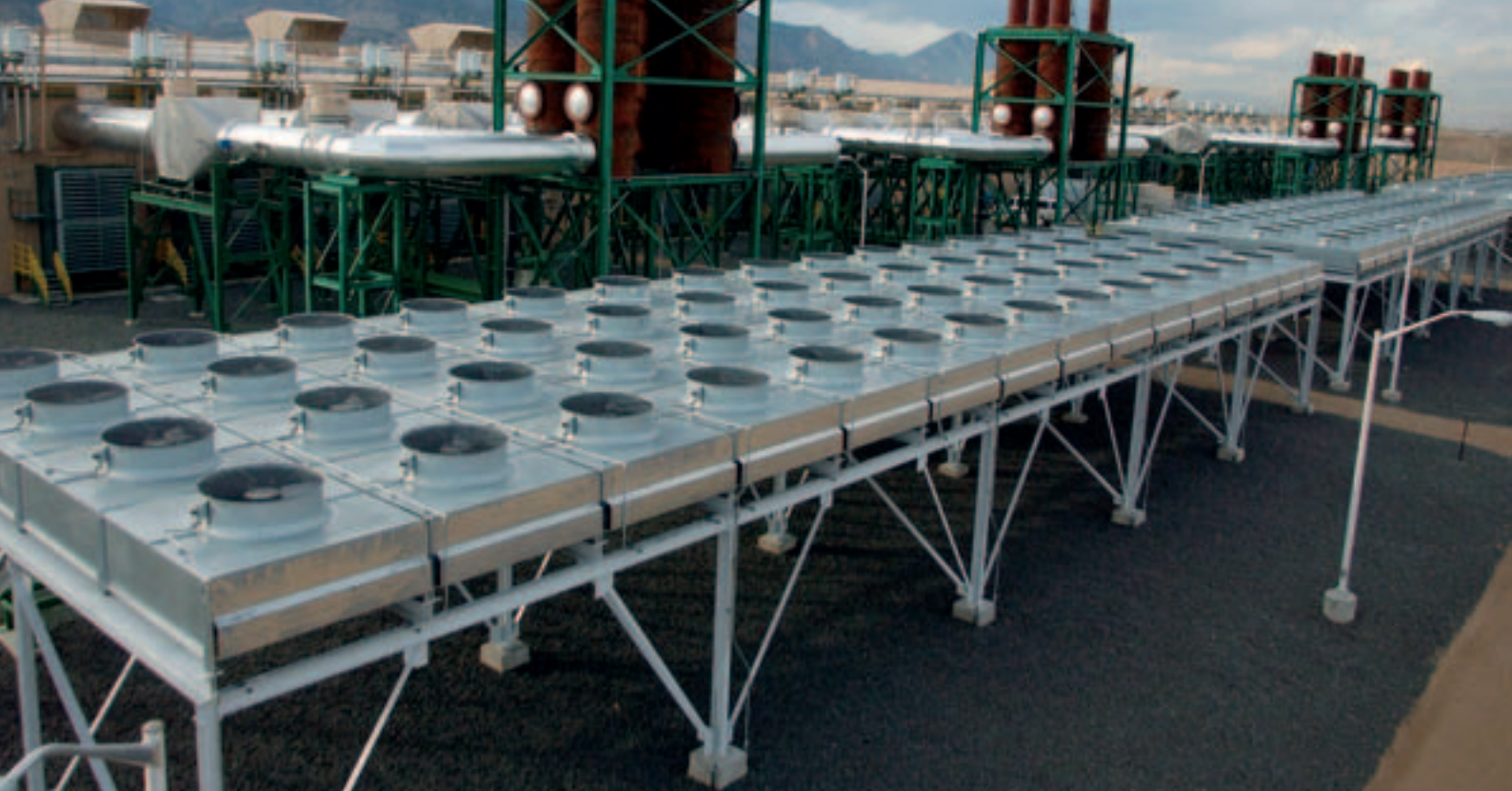
Plains End power plant (111 MW) uses ULE-type SCR (Selective Catalytic Reduction) and oxidation catalysts.
