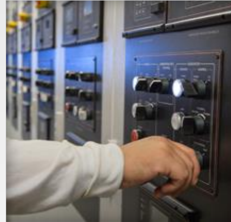
Electrical and Automation services
