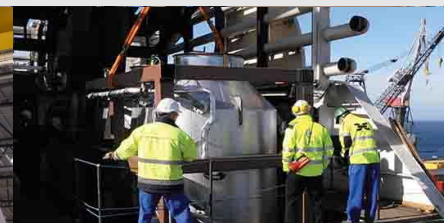
EXHAUST GAS CLEANING
