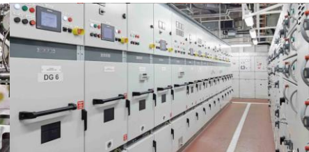
POWER ELECTRIC SYSTEMS
