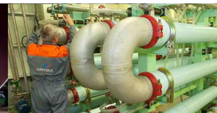
WASTE, OIL & FRESH WATER MANAGEMENT
